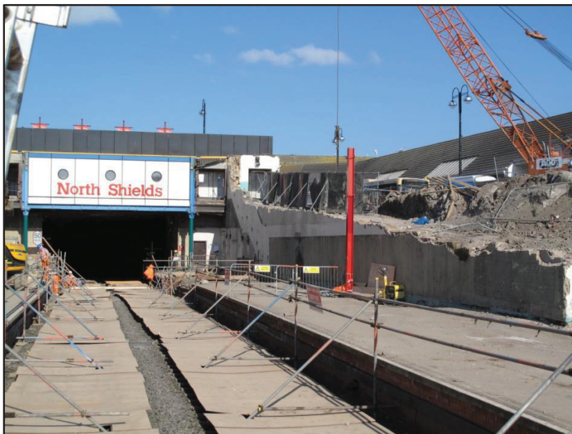
7) North Shields showing demolition of the Platform 2 ramp and foundations. The railway tracks are covered over for their own protection and overhead power lines have been taken down to allow work to take place.
