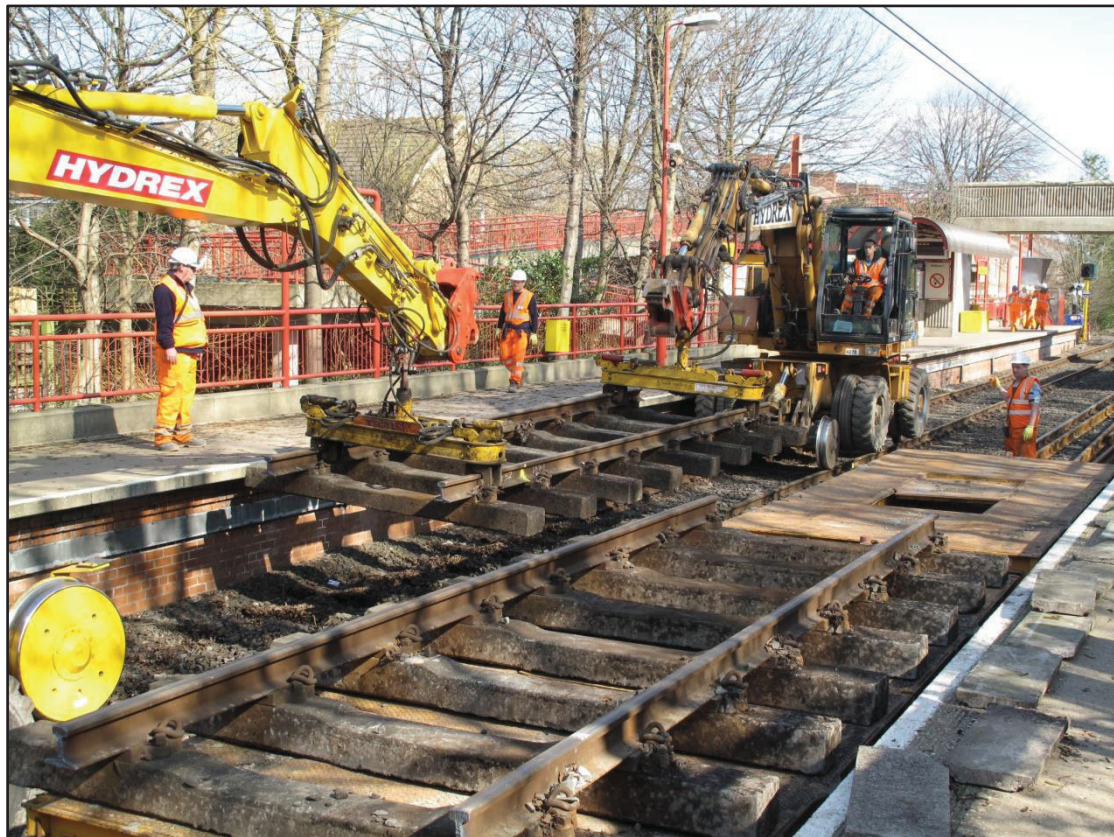
4) Old sections of track are lifted out in one piece at Hadrian Road
