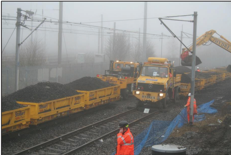
5) Old ballast is carried by rail vehicle to the Chillingham Road site compound, for removal to lorry.
