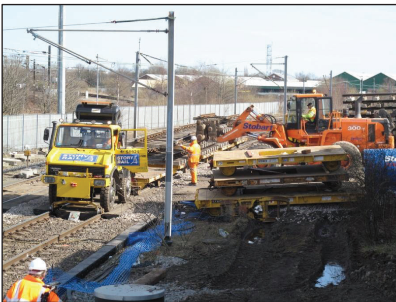
6) Redundant track is unloaded from rail vehicles at Chillingham Road site compound for removal by lorry,
